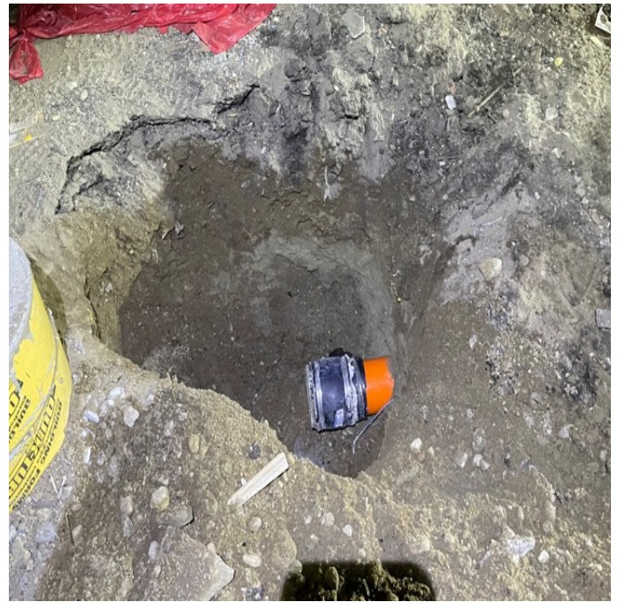
Attempted repair done by the contractor. The contractor capped the main and then use hose clamps to keep the cap in place.
