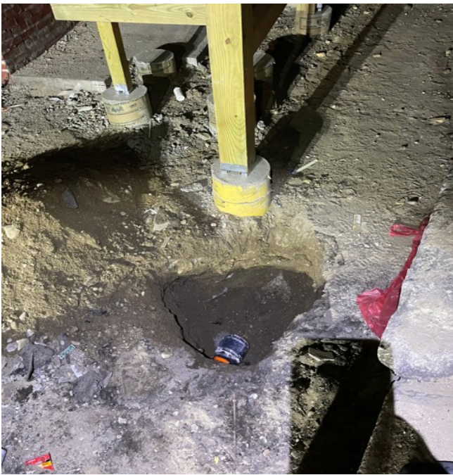
Damage location. No markings existed as no CBYD ticket was called in.
